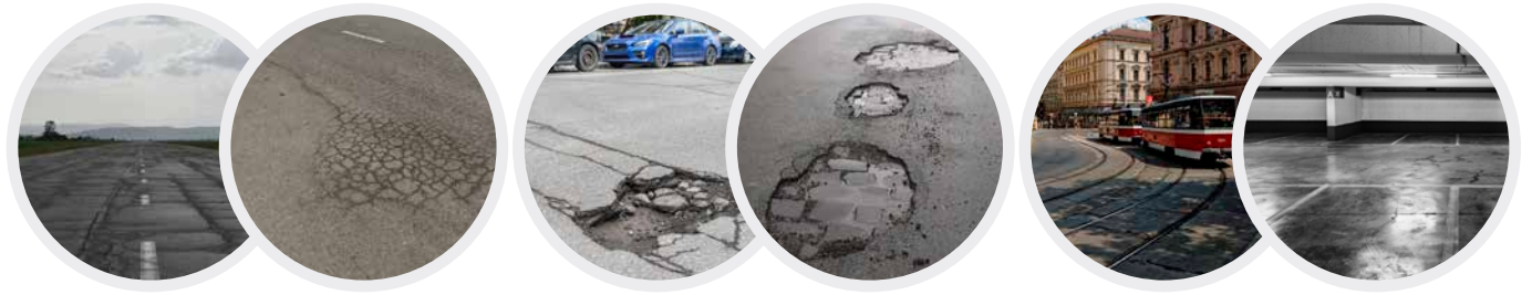
Example of cracking for area-wide repairs
